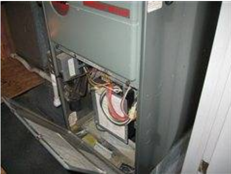
Photo 43 Service panel Maximum air temperature at register nearest unit: 118 degrees F Maximum air temperature at remote register: 120 degrees F
