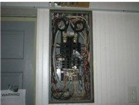
Photo 8 Main panel- cover removed
